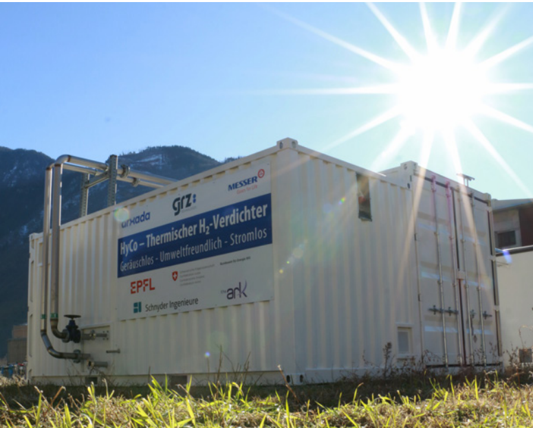
CH-030: Industrial-Scale Metal Hydrides Hydrogen Compressor HyCo
